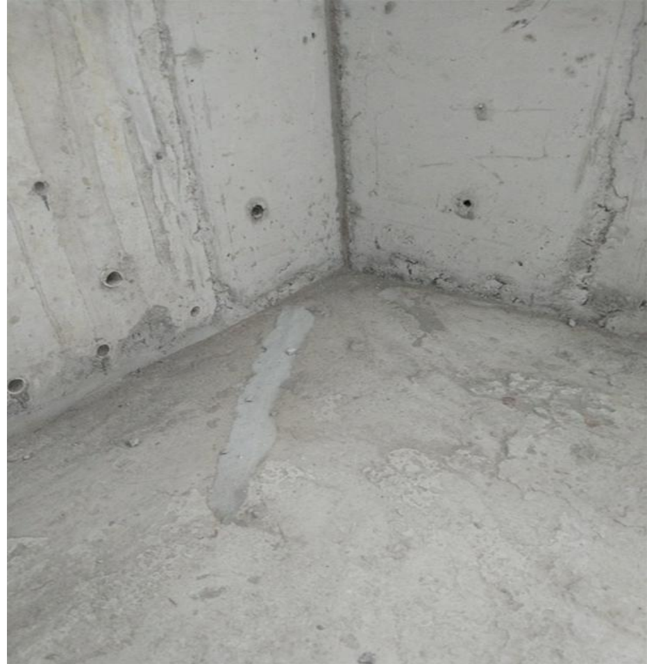
阳台悬挑构件露筋
